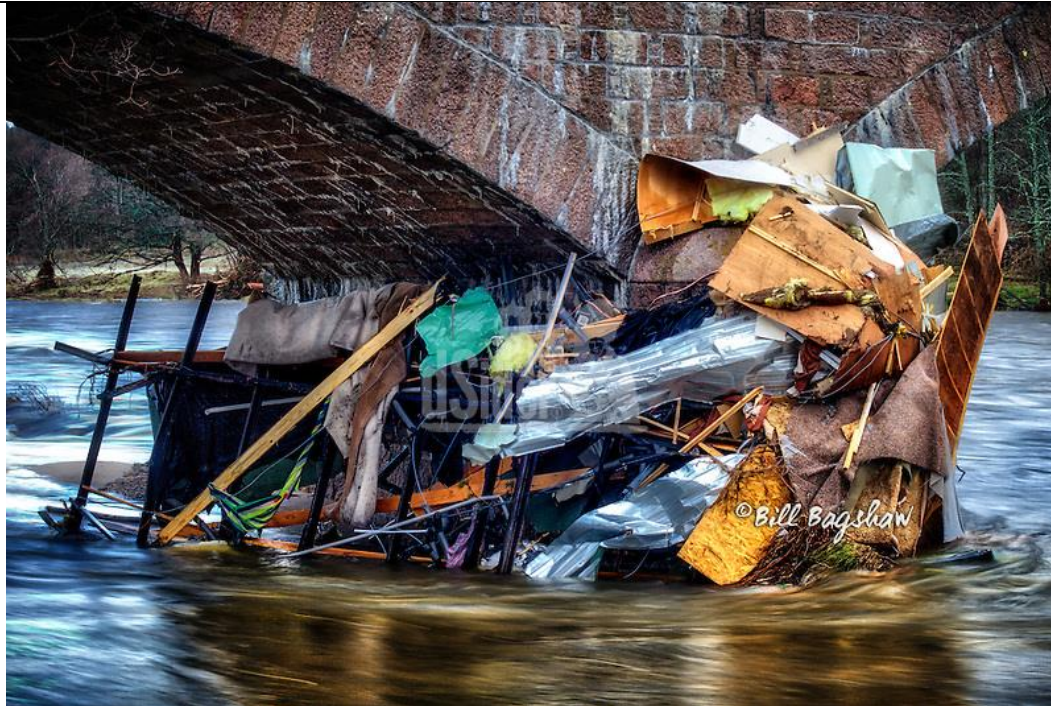
Photo 9: The Bridge after the Flood showing debris – which would restrict flow
